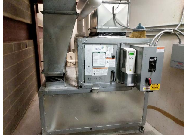
Photo #16 Typical Auditorium Air Handling Unit
