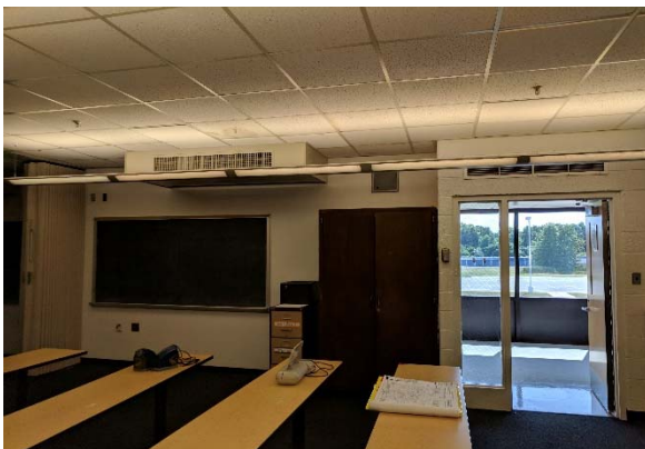
Photo #17 Typical Classroom Horizontal Unit Ventilator
