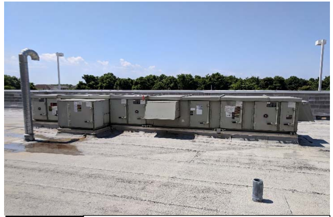
Photo #26 Typical Rooftop Air Handling Unit
