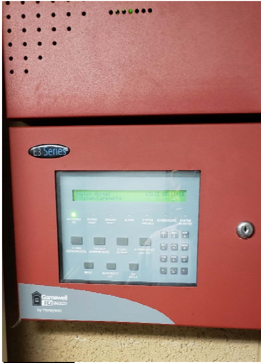
Photo #1 Fire Alarm Control Panel
