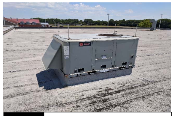
Photo #12 Typical Packaged DX Roof Top Unit
