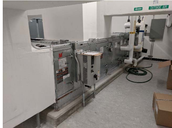
Photo #20 Typical Indoor Air Handling Unit
