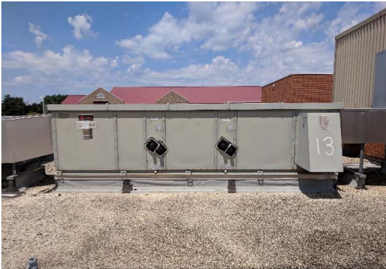
Photo #27 Typical Rooftop Energy Recovery Unit
