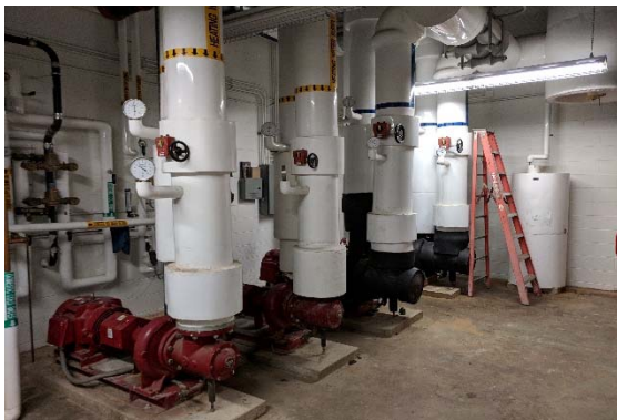
Photo #5 Area H Mechanical Room Secondary Heating and Cooling Pumps
