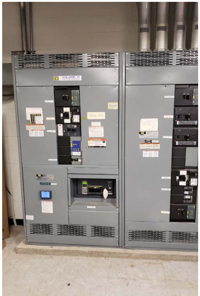
Photo #4 Switchboard MPS
