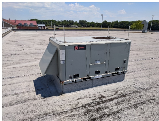
Photograph 3: Typical Packaged DX Unit
