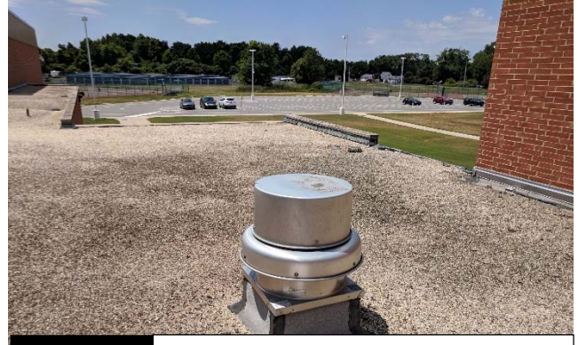
Photo #28 Typical Rooftop Exhaust Fan
