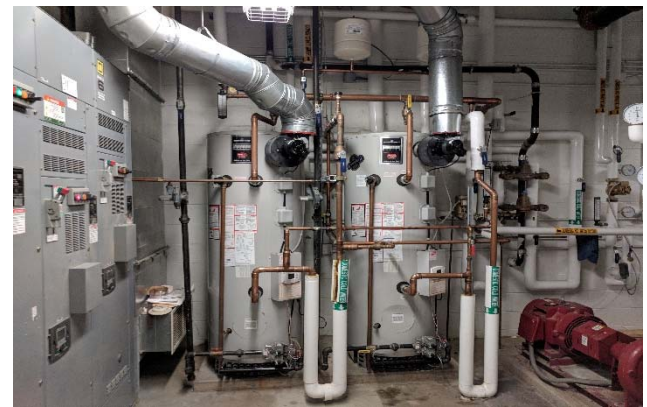
Photo #4 Area H Room Domestic Water Heaters
