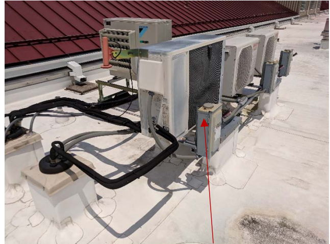
Photo #2 Disconnects on roof showing rust and wear
