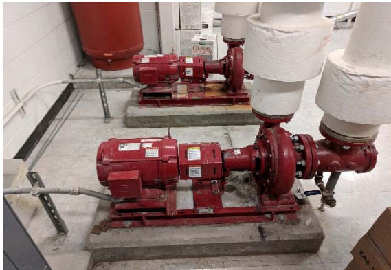
Photo #3 Area A Mechanical Room Secondary
