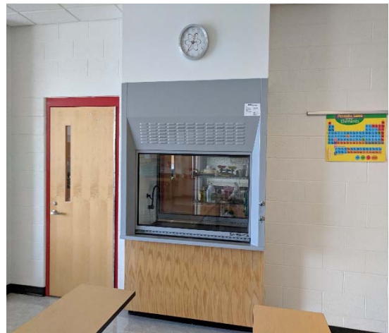
Photo #22 Typical Lab Exhaust Hood
