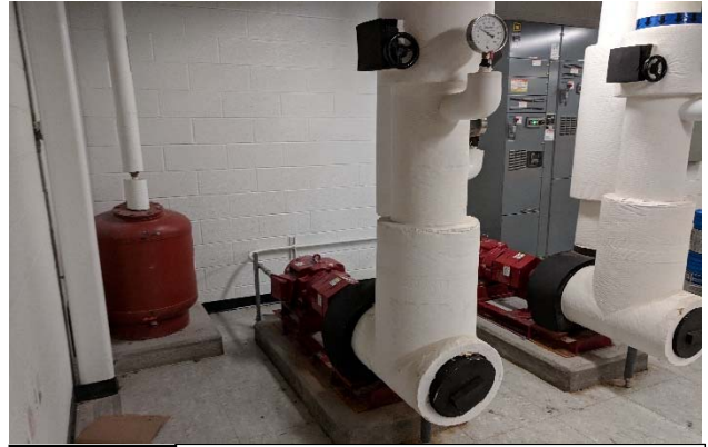
Photo #2 Area A Mechanical Room Secondary Chilled Water Pumps
