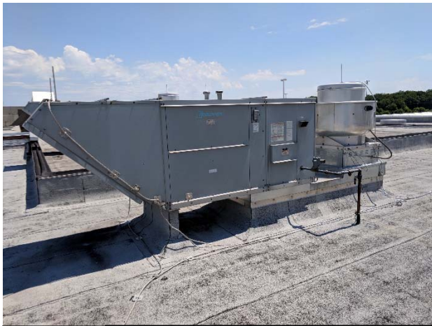
Photo #21 Typical Kitchen Make-Up Air Unit
