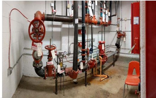
Photo #9 Fire Pump Room
