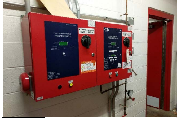
Photo #8 Fire Pump Controller
