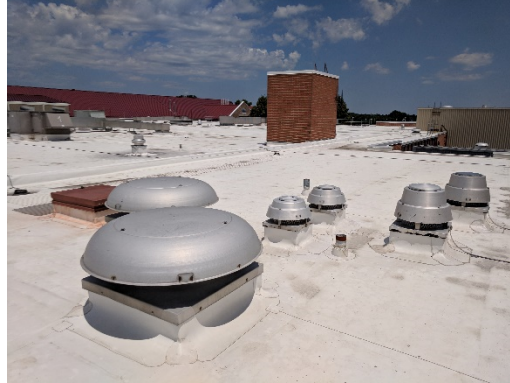
Photograph 4: Typical Rooftop Fans and Gravity Hoods
