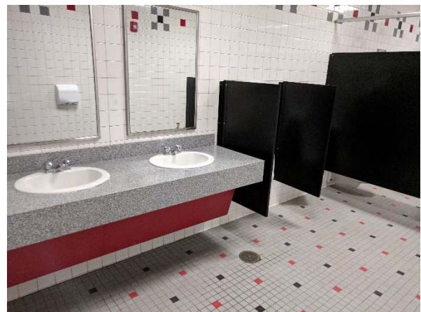
Photo #24 Typical Lavatory
