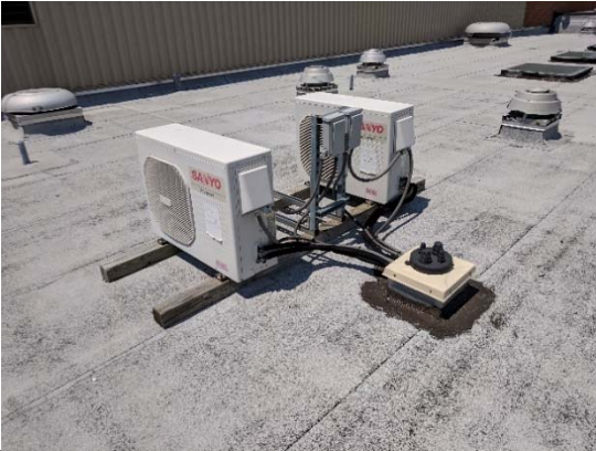
Photo #19 Typical DX Split System Condensing Units
