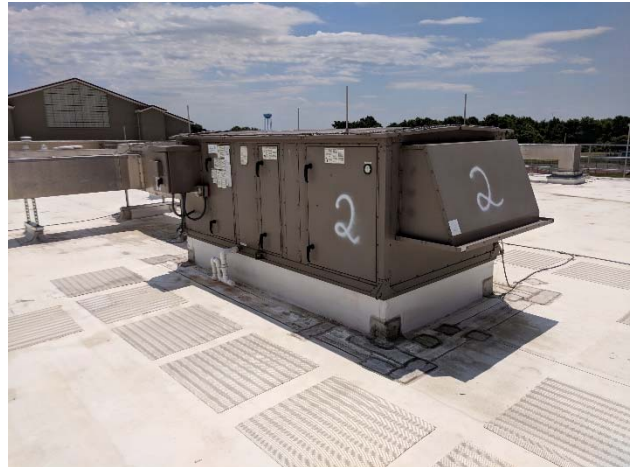
Photo #14 P-01.1 and P01.2 (RTU)
