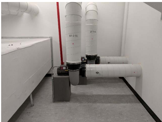
Photo #23 Typical Lab Hood Inline Exhaust Fans
