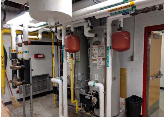
Photo #1 Area A Mechanical Room Domestic Water Heaters
