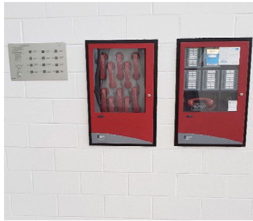
Photo #3 Lobby Annunciator Panel and Rescue Assistance
