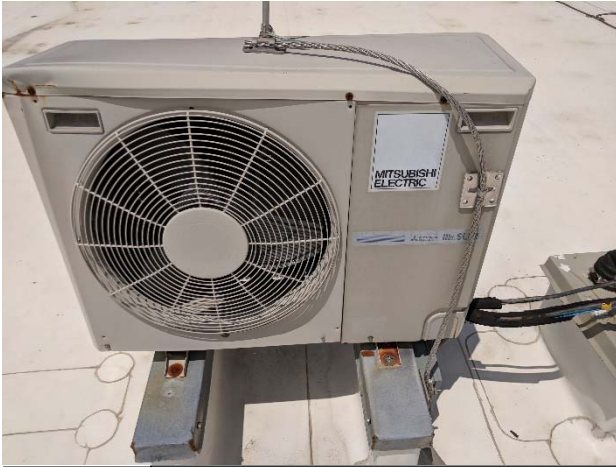
Photo #13 P-01 (Rooftop CU-P-01.5 with R-22)
