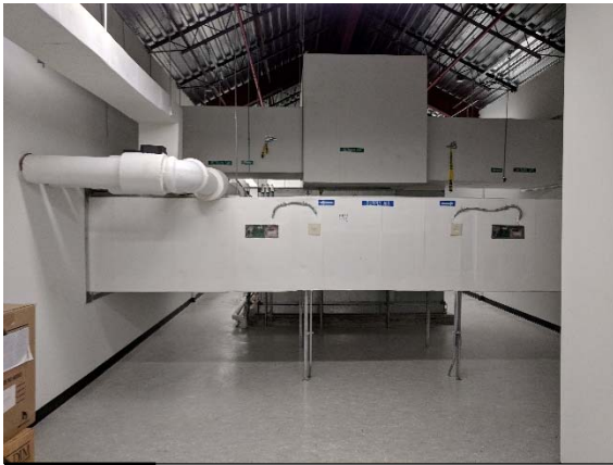
Photo #25 Typical Mechanical Mezzanine
