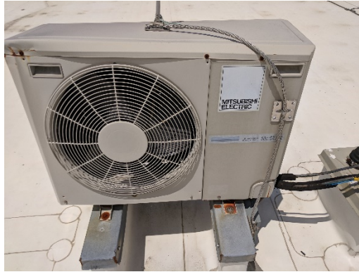
Photograph 2: Unlabeled Split DX Unit with R-22
