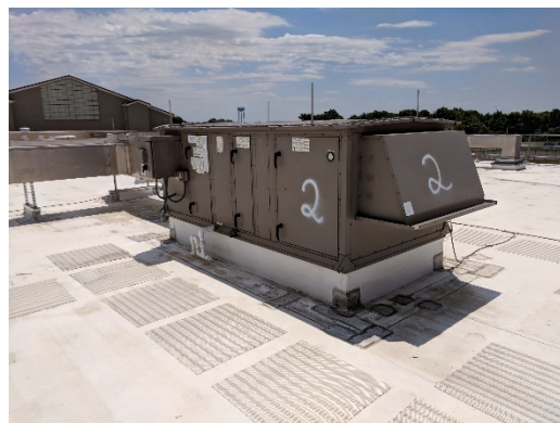
Photograph 1: Typical Existing RTU
