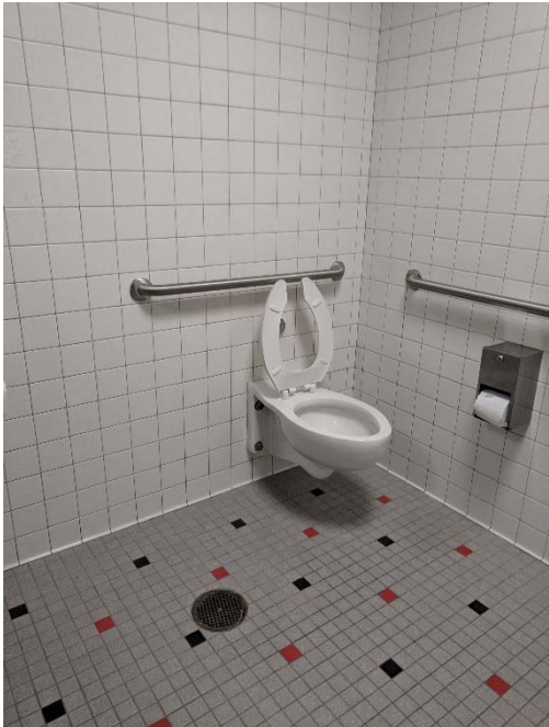
Photo #31 Typical Water Closet
