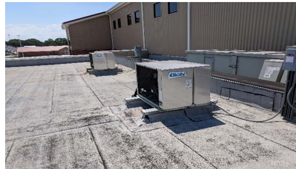
Photo #10 Kitchen Refrigeration Condensing Units
