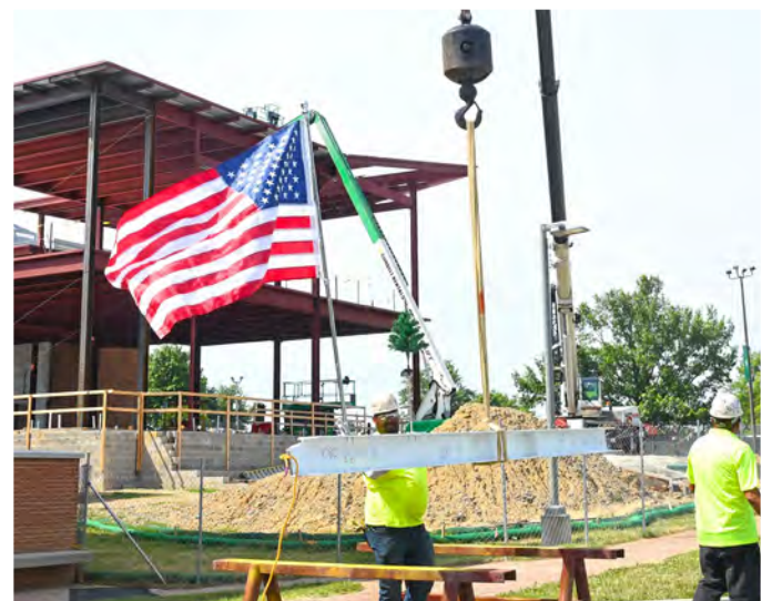
An American flag is raised to commemorate the final beam being placed atop the Stanton Campus culinary arts expansion project.
