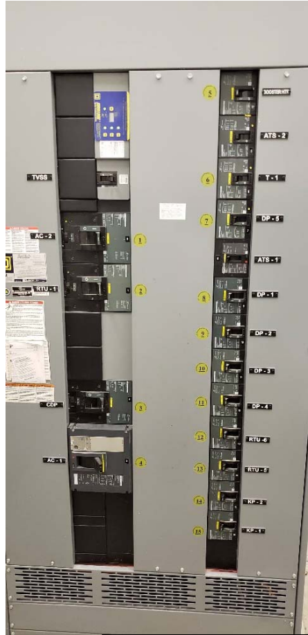
Photo #6 Distribution Section of Main Switchboard
