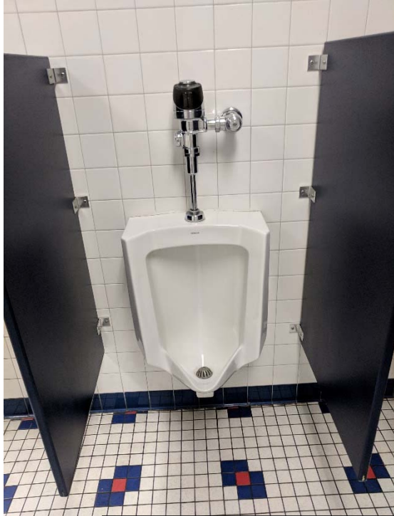
Photo #13 Typical Urinal
