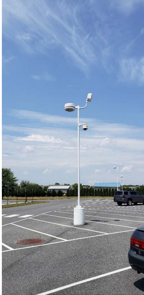
Photo #14 Typical Parking Lot Light Fixture
