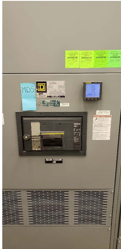
Photo #2 2500A Breaker in Main Switchboard
