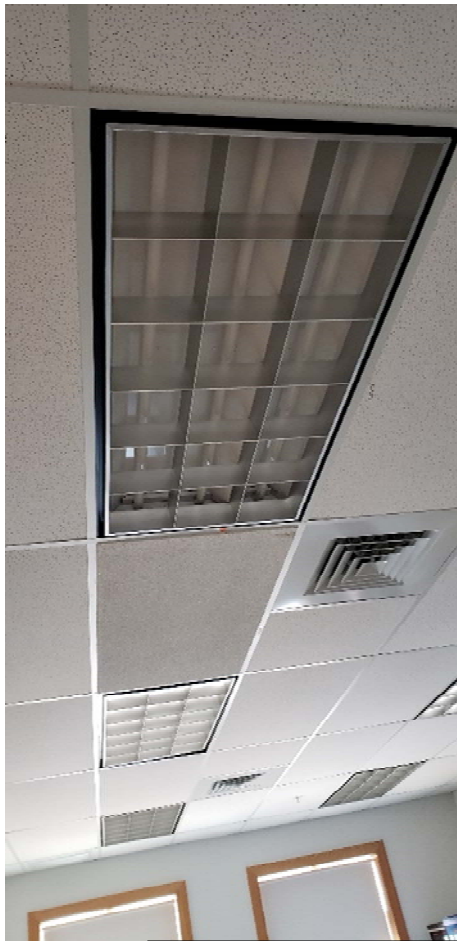
Photo #11 Typical Classroom Lighting Fixture
