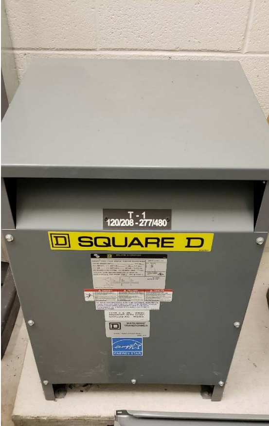
Photo #1 208V to 480V Boost Transformer
