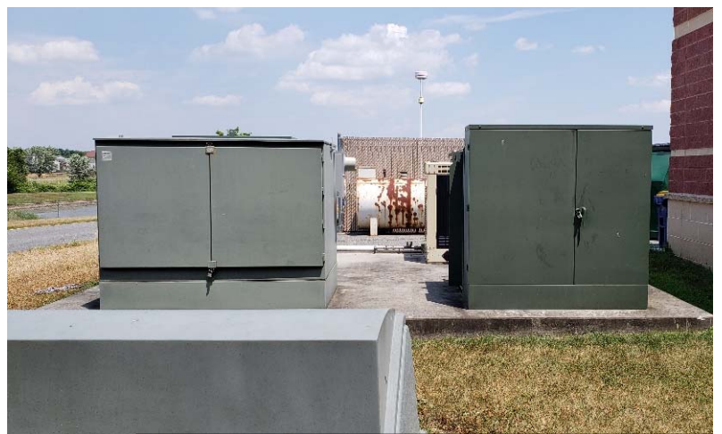
Photo #9 Metering Station, Transformer PMH-5 Switch and Generator
