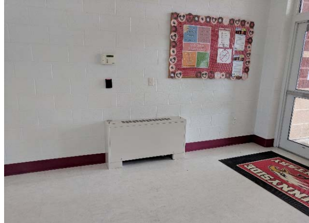
Photo #14 Typical Vestibule Cabinet Heater
