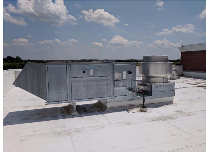
Photo #6 Kitchen Make Up Air Unit
