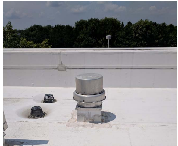
Photo #10 Typical Rooftop Exhaust Fan
