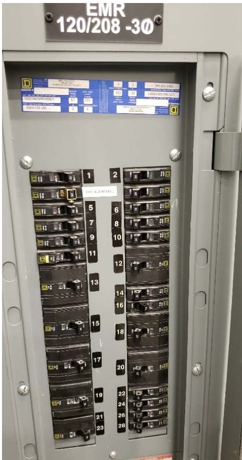
Photo #19 Typical Square D NQOD Branch Panelboard
