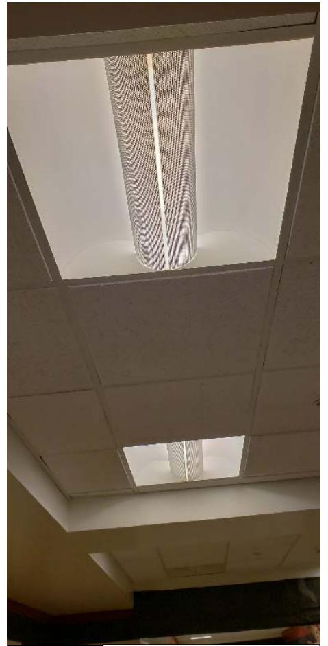
Photo #12 Typical Corridor Lighting Fixture
