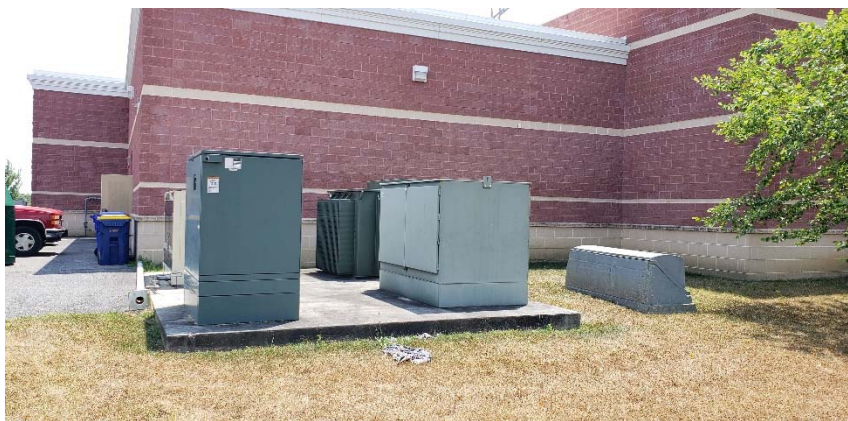
Photo #4 Exterior Electrical Equipment and Wallpack
