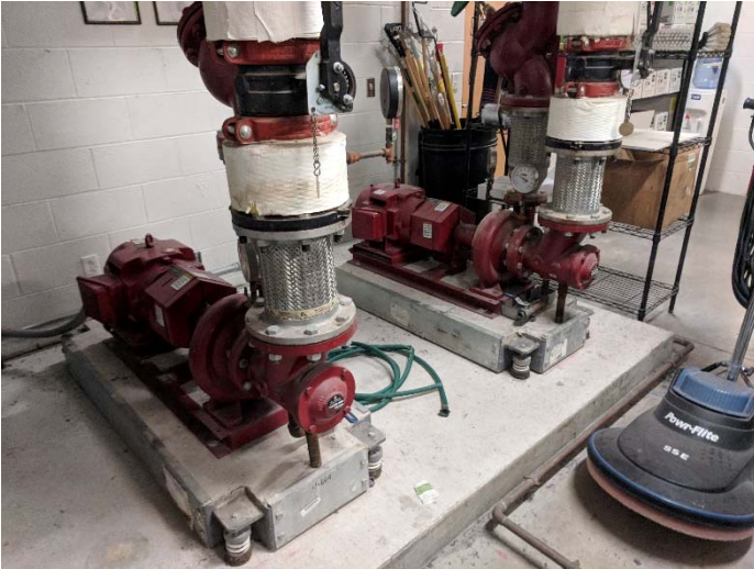
Photo #5 Heating Water Pumps in Mechanical Room
