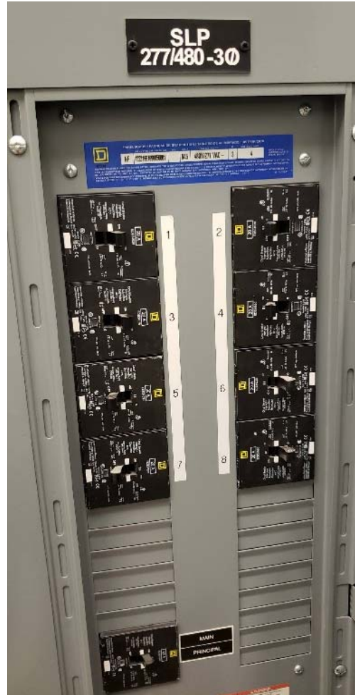
Photo #18 Typical Square D NF (480V) Branch Panelboard
