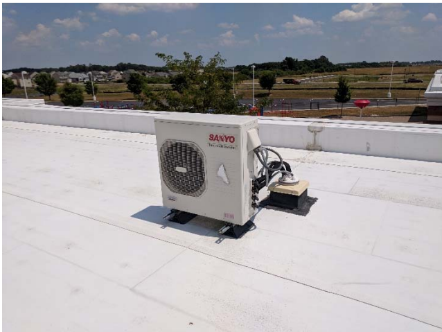
Photo #11 Typical Split DX Condensing Unit
