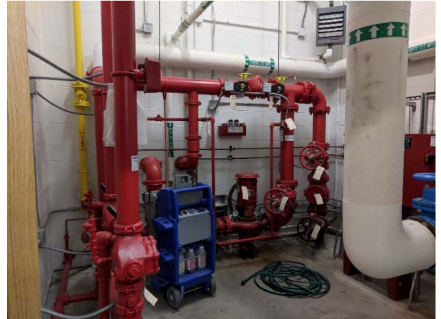
Photo #2 Domestic and Fire Protection Water Entrances
