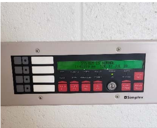
Photo #8 Fire Alarm Annunciator Panel
