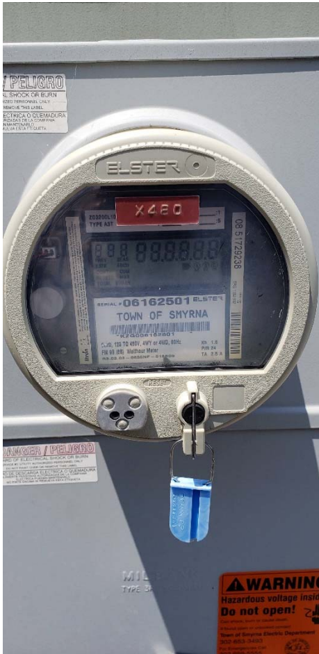
Photo #10 Primary Meter located on Metering Station
