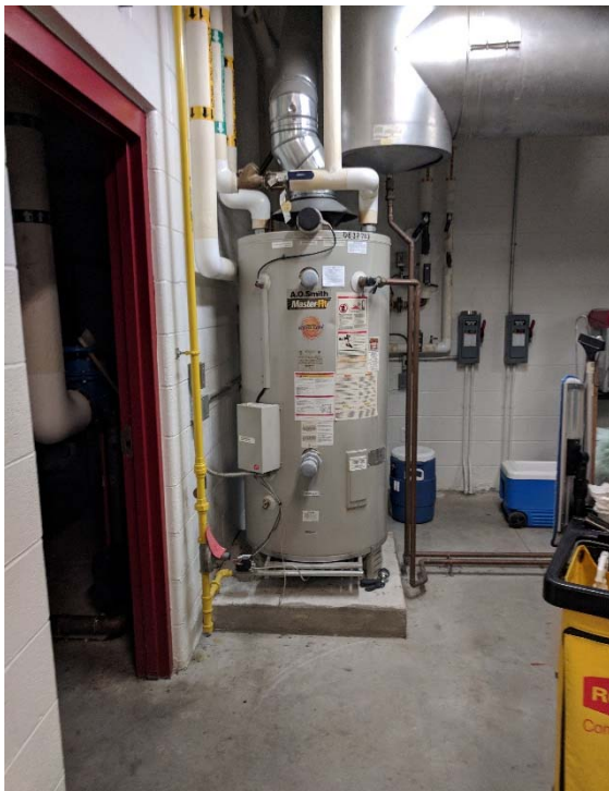
Photo #3 Domestic Water Heater
