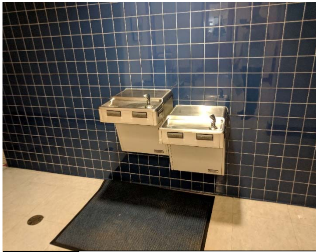
Photo #15 Typical Electric Water Coolers
