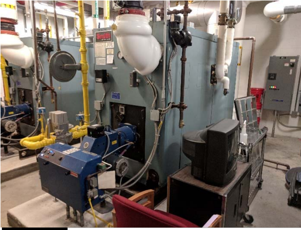
Photo #1 Boilers in Mechanical Room
