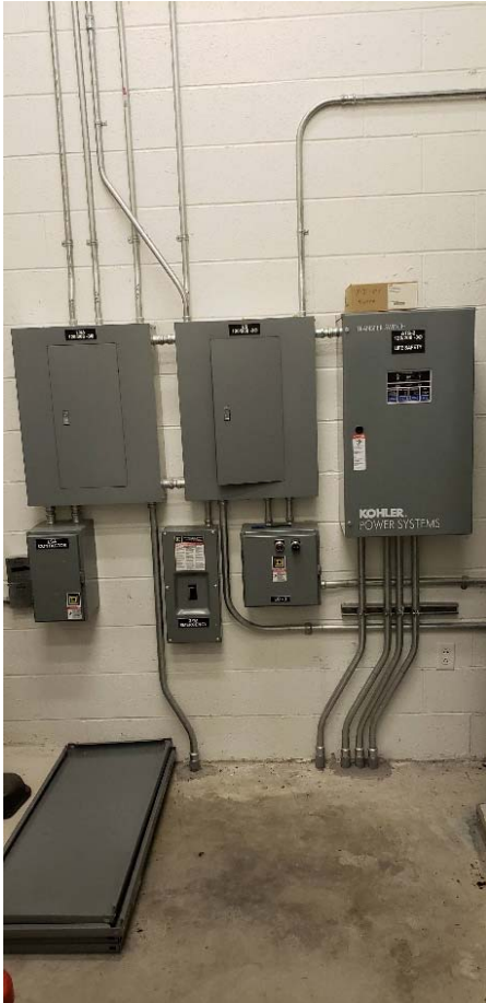
Photo #5 ATS-2 and Life Safety Panelboards
