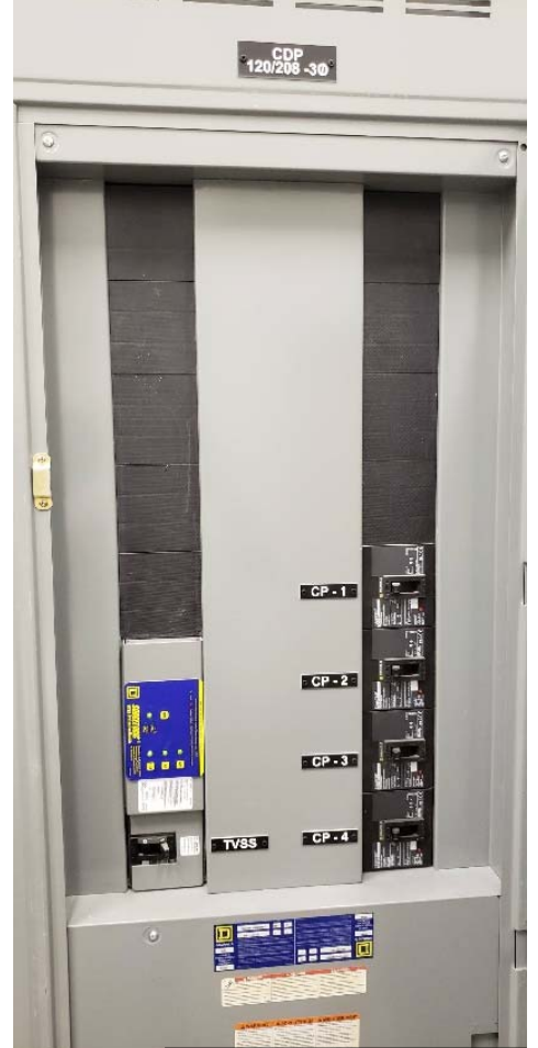
Photo #15 Typical Square D HCM Distribution Panelboard
