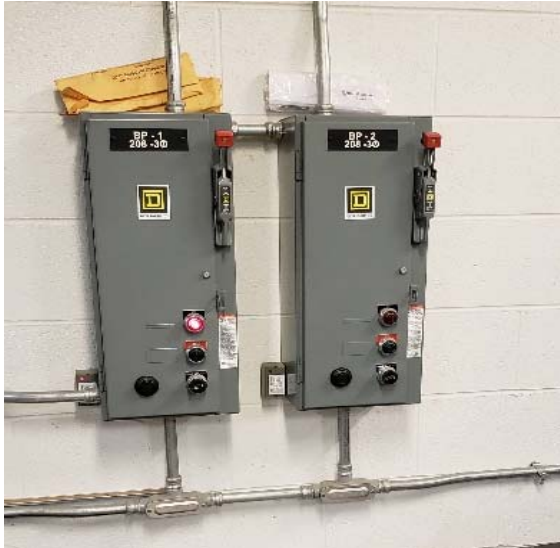
Photo #17 Typical Square D Motor Controllers
