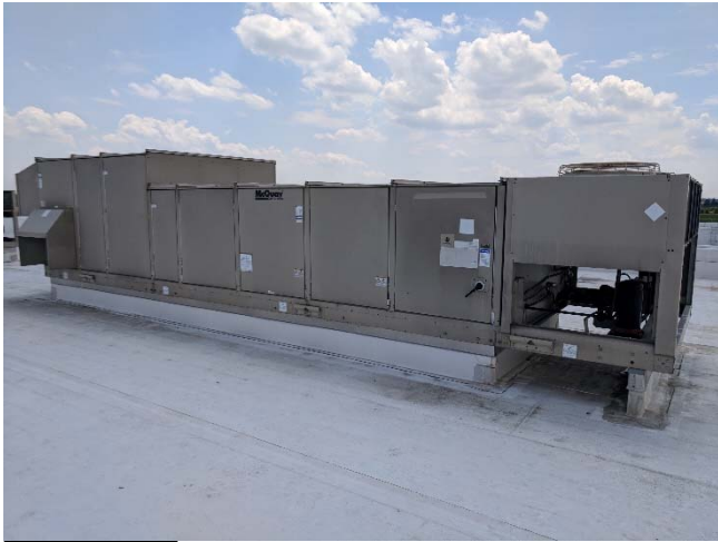
Photo #9 Typical Packaged RTU with Energy Recovery
