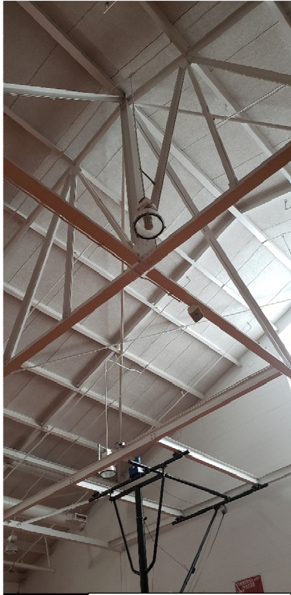
Photo #9 Gym Light Replaced with LED lamp
