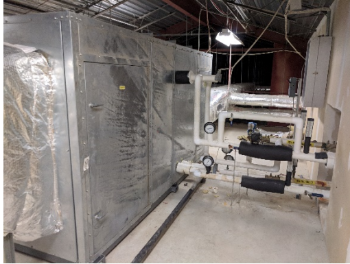
Photograph 2: ERU-2 in Mechanical Mezzanine
