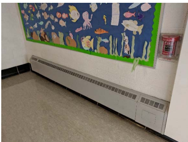
Photo #15 Typical Finned Tube Radiator
