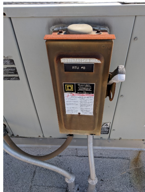
Photo #12 Exterior Disconnect Switch that needs to be replaced
