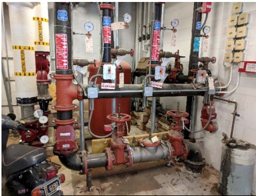
Photo #3 Fire Protection Zone Piping and Backflow Preventer
