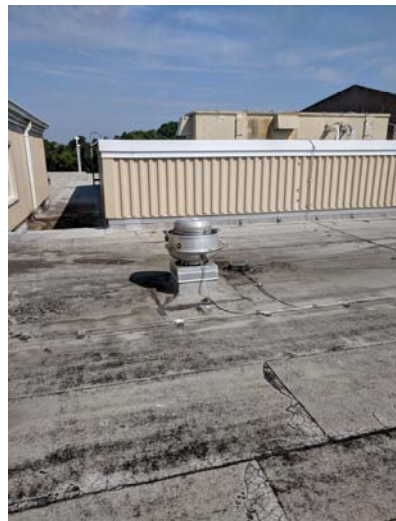
Photo #22 Typical Rooftop Exhaust Fan
