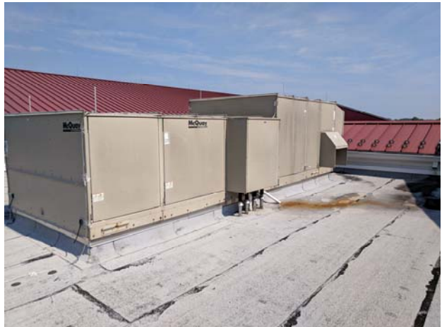
Photo #24 Typical Rooftop ERU
