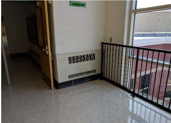
Photo #17 Typical Cabinet Heater
