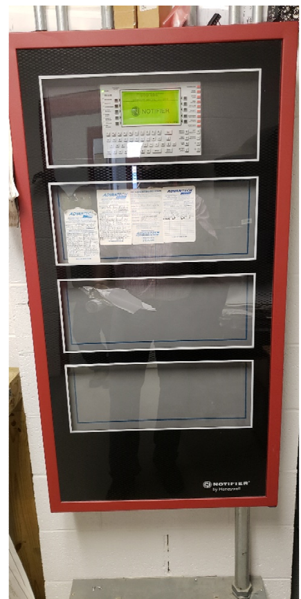
Photo #7 Fire Alarm Control Panel
