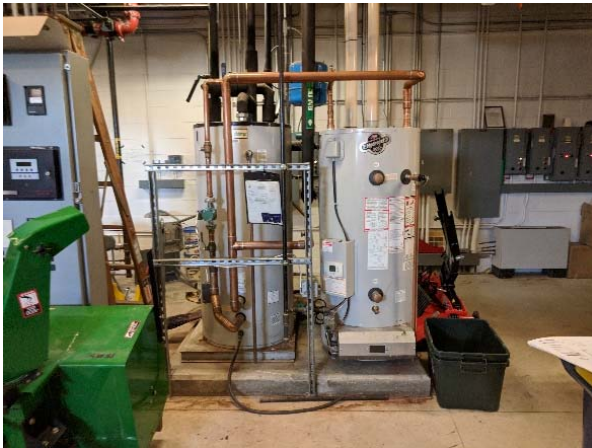
Photo #5 Domestic Hot Water Heaters
