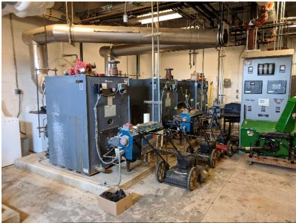
Photo #7 Abandoned Boilers
