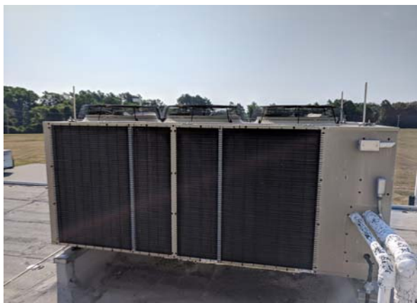
Photo #27 CU-2a Typical Split DX Outdoor Condensing Unit
