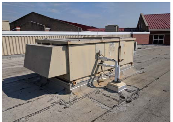
Photo #28 Typical 4-Pipe RTU
