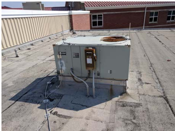
Photo #21 Typical RTU
