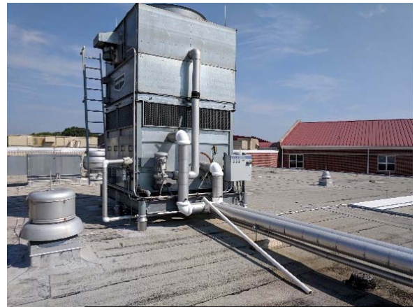
Photo #14 Abandoned Closed Circuit Cooler
