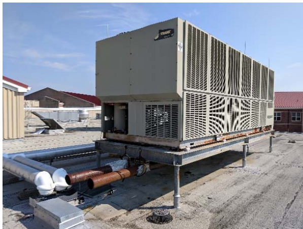
Photo #19 Abandoned Air Cooled Chiller
