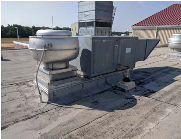
Photo #23 Typical Kitchen Ventilation Unit
