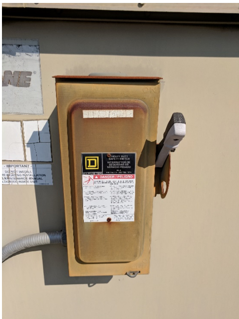
Photo #11 Exterior Disconnect Switch that needs to be replaced
