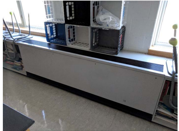
Photo #12 Typical Vertical Unit Ventilator
