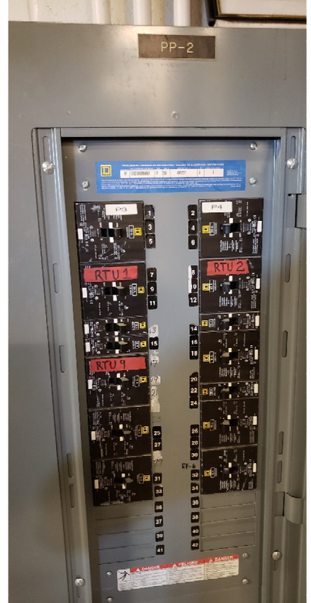
Photo #3 Typical Square D Branch Panelboard
