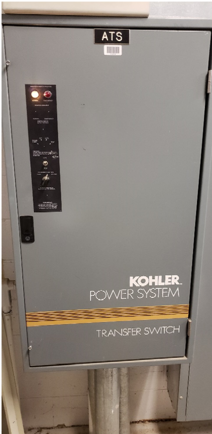
Photo #5 Automatic Transfer Switch
