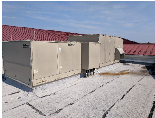
Photograph 1: ERU-5 on Roof
