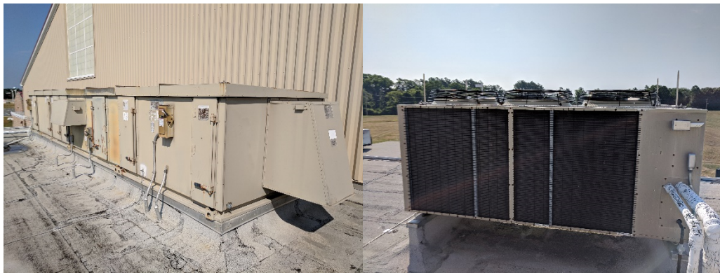
Photograph 3: Typical Rooftop Unit Split System
