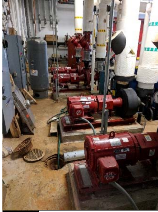
Photo #2 Secondary Heating and Cooling Pumps
