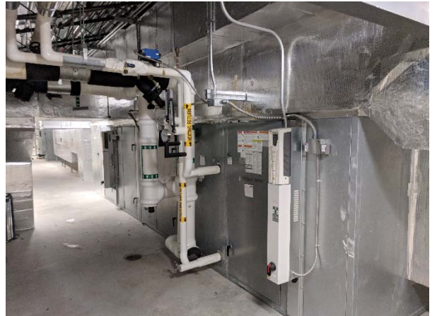
Photo #8 Typical Indoor AHU in Mechanical Mezzanine
