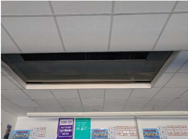
Photo #11 Typical Horizontal Unit Ventilator
