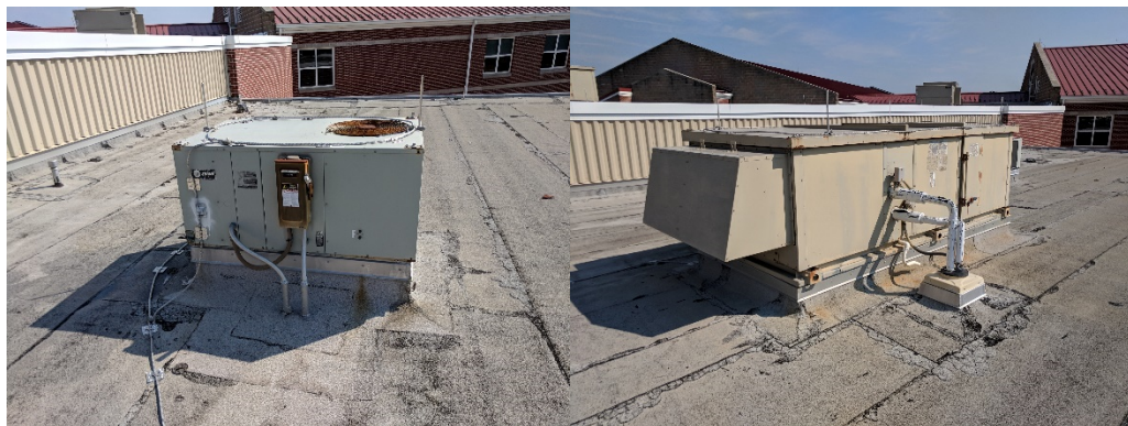
Photograph 4: Typical RTUs on Roof
