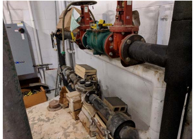
Photo #6 Domestic Water Entrance
