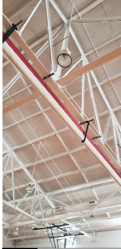
Photo #10 Gym Light with Metal Halide Lamp
