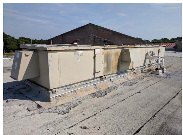
Photo #16 Typical 4-Pipe Rooftop Air Handling Unit
